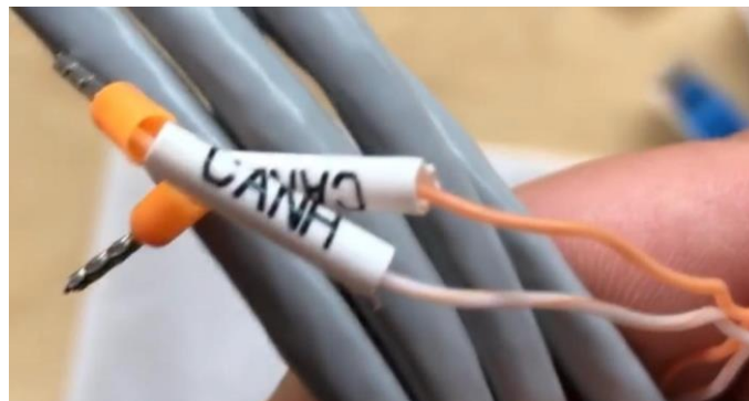
Figure 47 - Inverter/HV BOX communication cable
