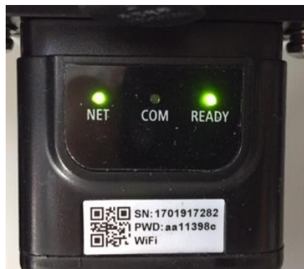
Figure 135 - Irregular communication status between inverter and adapter
