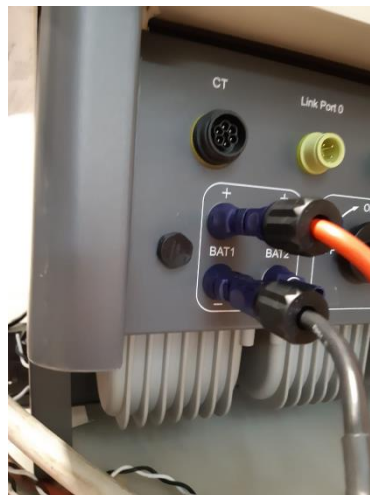
Figure 24 - Inverter-side DC power connection with a single battery input populated
