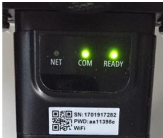
Figure 130 - Irregular communication status between the adapter and remote server
