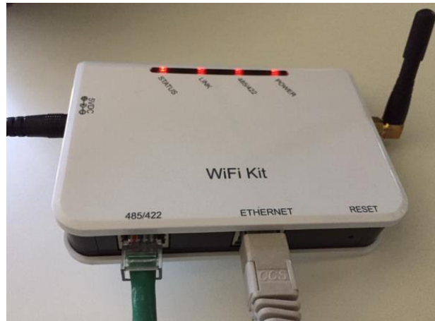
Figure 144 – Ethernet cable connected to the datalogger
