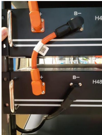
Figure 21 - Power connection (negative) between the BMS and the last battery module
