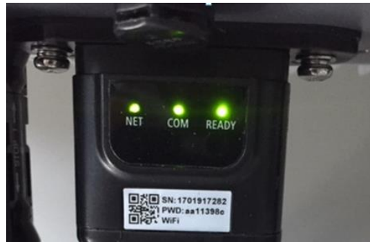
Figure 134 - Final status of LEDs
