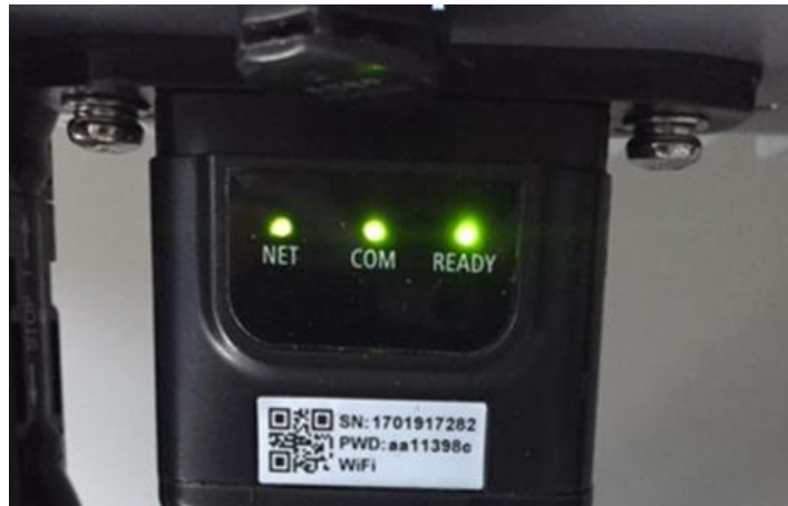
Figure 128 - Final status of LEDs
