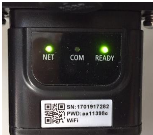
Figure 129 - Irregular communication status between the inverter and adapter
