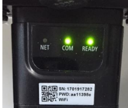
Figure 136 - Irregular communication status between the adapter and remote server
