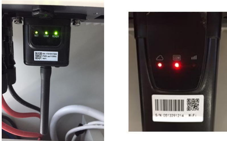
Figure 116 - Final status of LEDs
