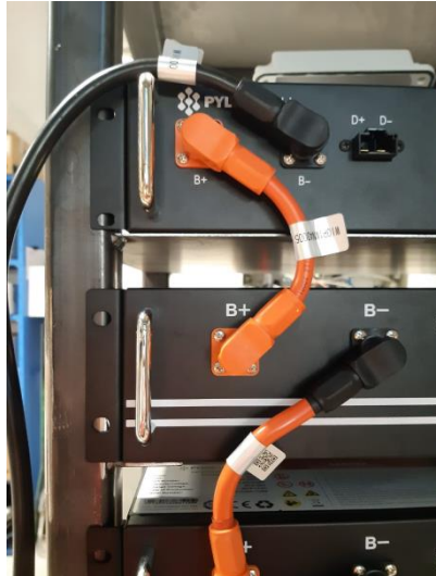
Figure 20 - Power connection (positive) between the BMS and first battery module
