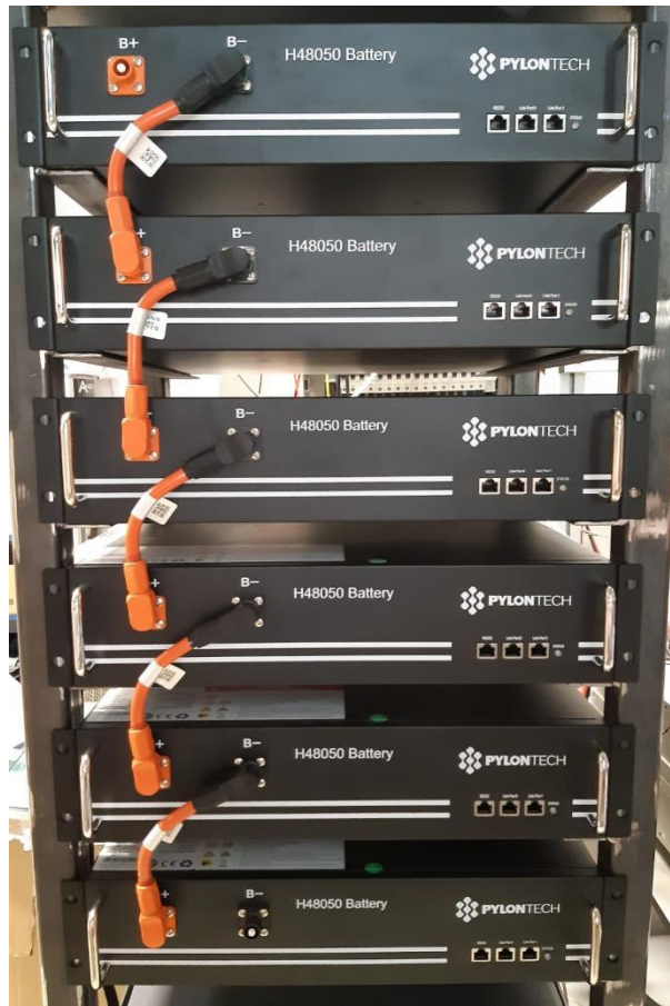
Figure 18 - Power cable between battery modules
