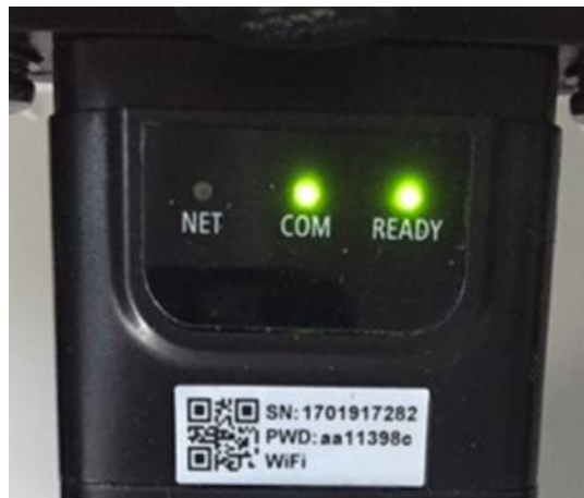
Figure 67 - Irregular communication status between the adapter and remote server
