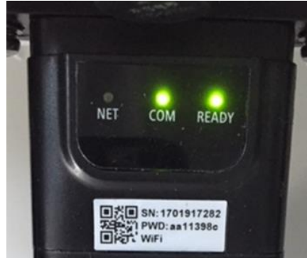
Figure 73 - Irregular communication status between the adapter and remote server
