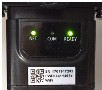
Figure 72 - Irregular communication status between inverter and adapter
