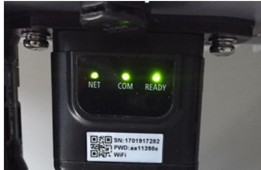
Figure 71 - Final status of LEDs
