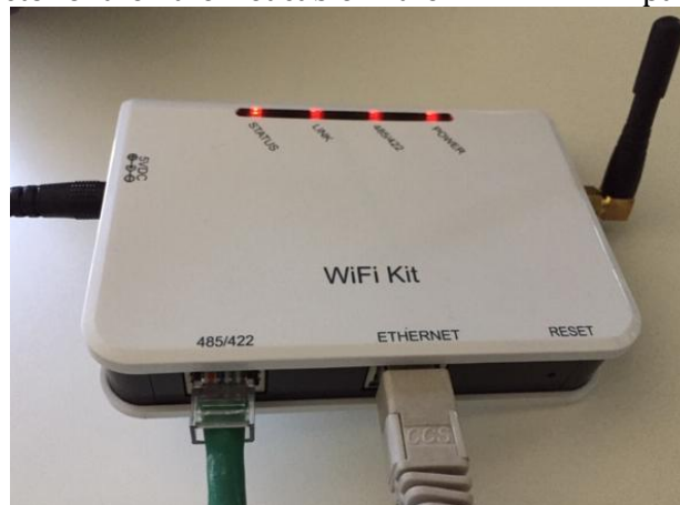
Figure 81 – Ethernet cable connected to the datalogger
