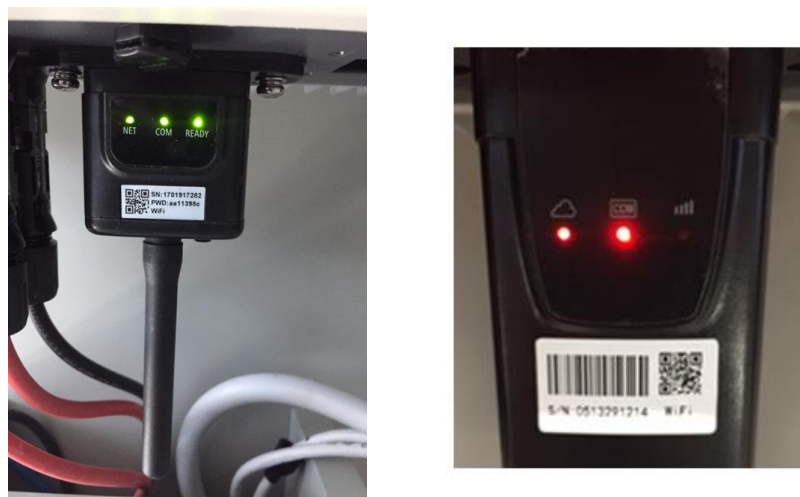
Figure 52 - Final status of LEDs
