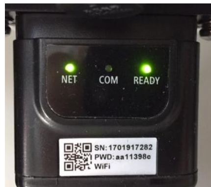
Figure 71 - Irregular communication status between inverter and adapter
