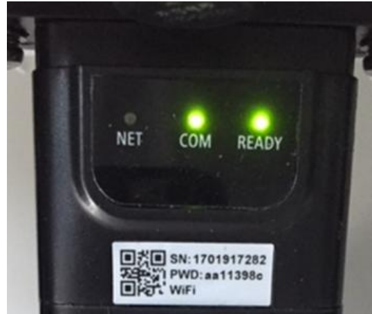
Figure 66 - Irregular communication status between the adapter and remote server
