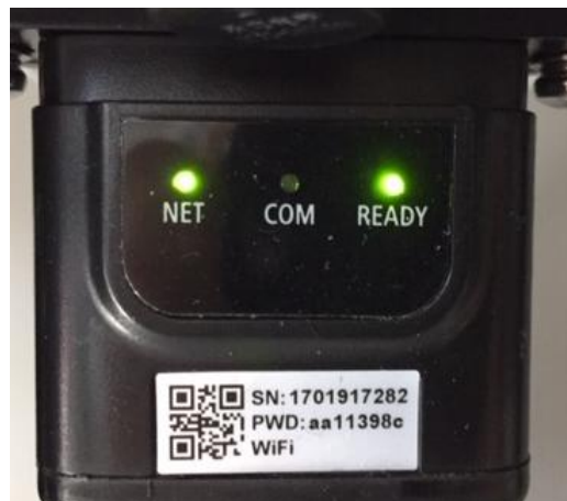
Figure 65 - Irregular communication status between the inverter and adapter
