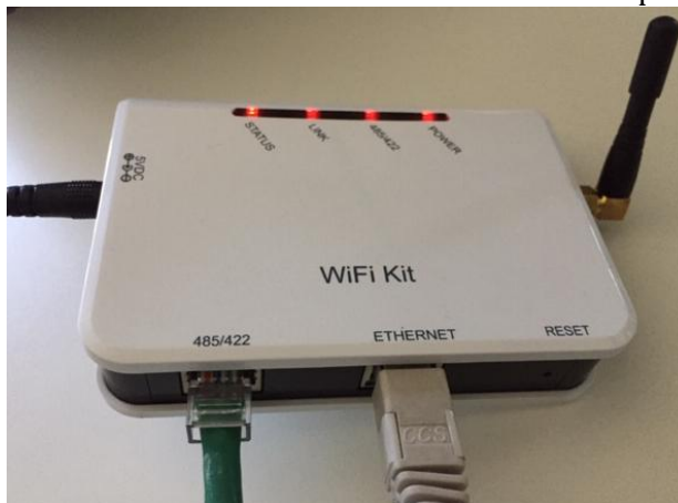
Figure 89 – Ethernet cable connected to the datalogger
