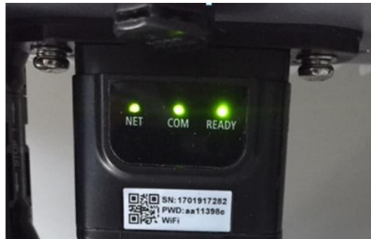
Figure 78 - Final status of LEDs
