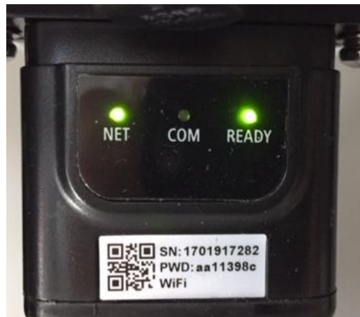
Figure 73 - Irregular communication status between the inverter and adapter
