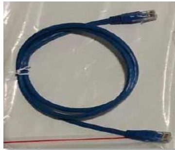
Figure 31 – Communication cable between WeCo 5k3 batteries
