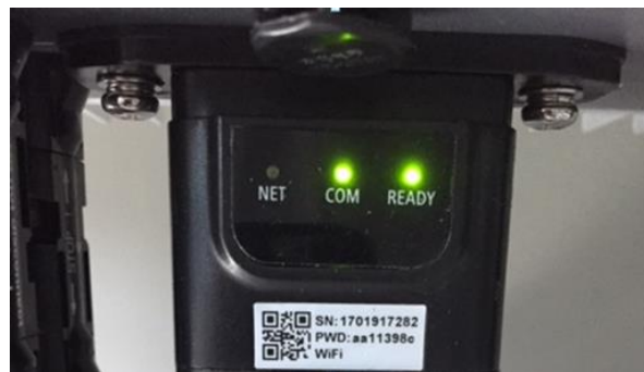
Figure 124 - Initial status of LEDs
