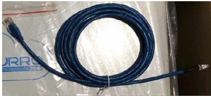
Figure 29 - Communication cable between the inverter and WeCo 5k3 battery
