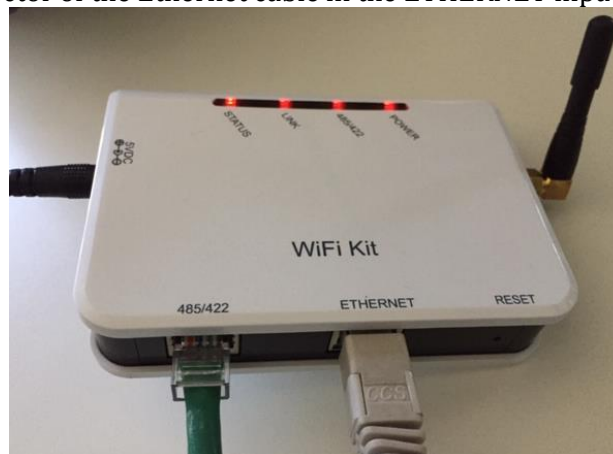
Figure 136 – Ethernet cable connected to the datalogger
