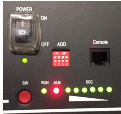
Figure 55 – Battery status after setting the POWER switch to ON and pressing the SW button
