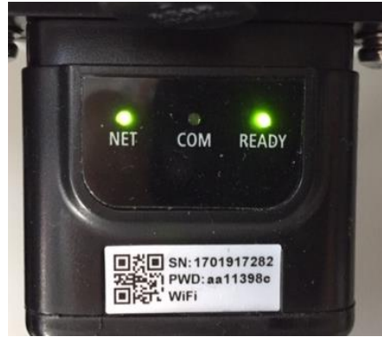
Figure 96 - Irregular communication status between inverter and adapter
