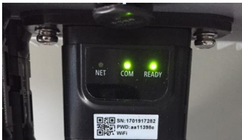
Figure 88 - Initial status of LEDs
