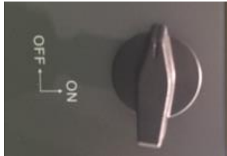
Figure 53 - Photovoltaic disconnecting switch
