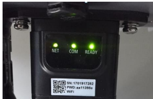
Figure 95 - Final status of LEDs
