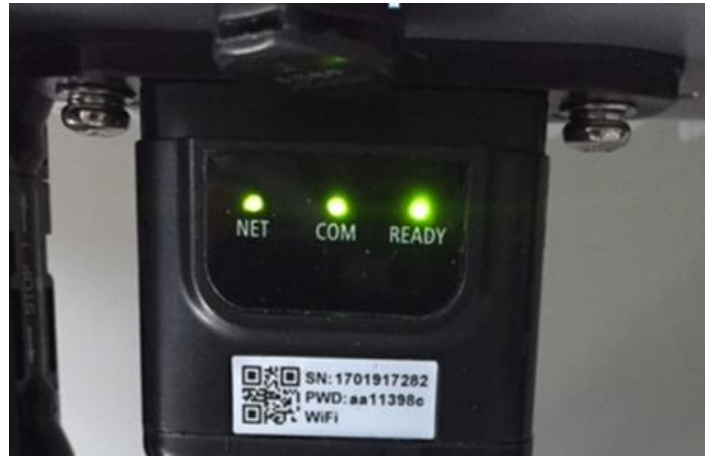
Figure 89 - Final status of LEDs
