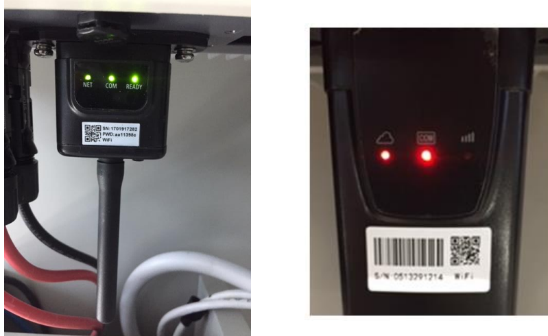
Figure 91 - Final status of LEDs
