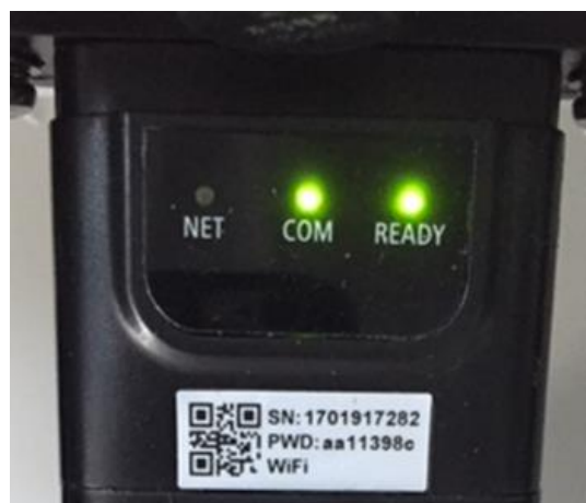
Figure 105 - Irregular communication status between the adapter and remote server
