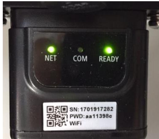
Figure 104 - Irregular communication status between the inverter and adapter
