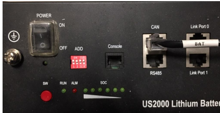
Figure 9 - Connecting the communication cable to the Pylontech battery
