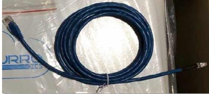
Figure 19 - Communication cable between the inverter and the WeCo 4k4 PRO battery
