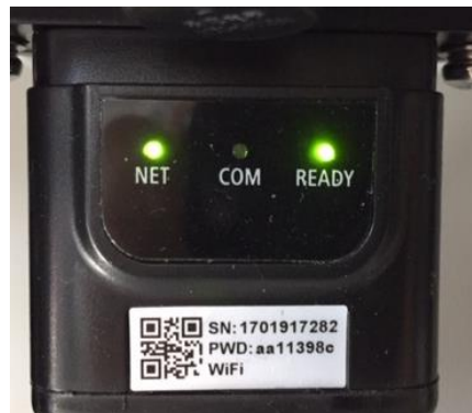
Figure 110 - Irregular communication status between inverter and adapter
