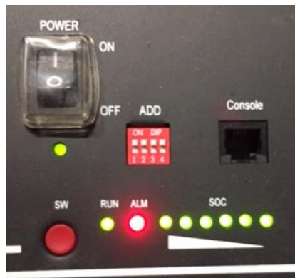
Figure 69 - Battery status after setting the POWER switch to ON and pressing the SW button
