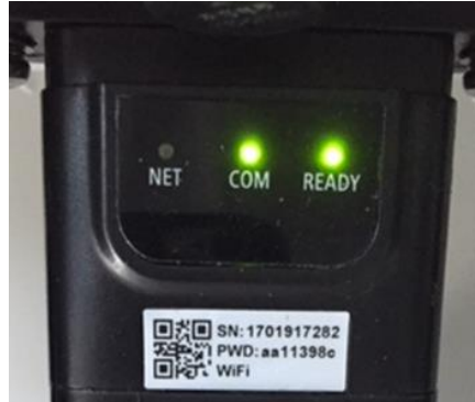
Figure 111 - Irregular communication status between the adapter and remote server
