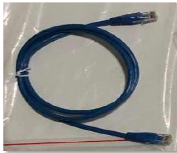
Figure 35 – Communication cable between WeCo 5K3XP batteries
